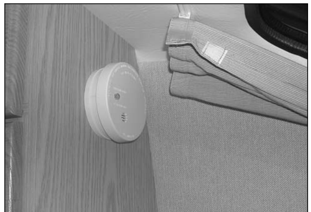
Picture F-P4: Smoke detector.
